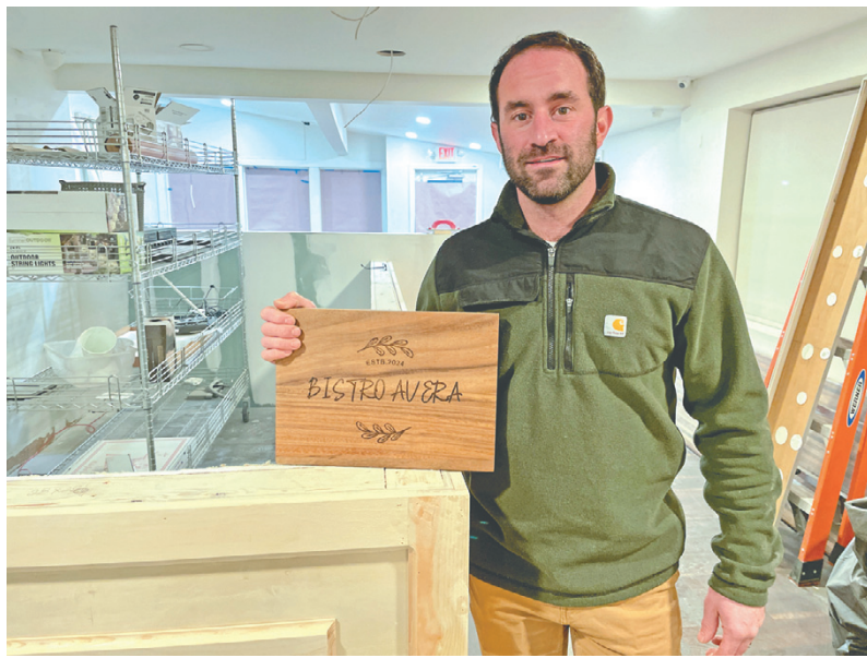
Chef Stephen Pusateri is preparing to open a second Lewiston restaurant, which he is calling Bistro Avera. Framing for a new bar was installed this week, and renovation work is well underway at 555 Center St.
